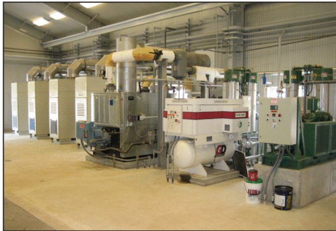
Four of nine compact Capstone C65-ICHP microturbines with exhaust heat recovery, shown in a facility designed by Basic Systems Inc. The nine microturbines provide all of the electrical power for a new compressor station at a remote gas storage site.
