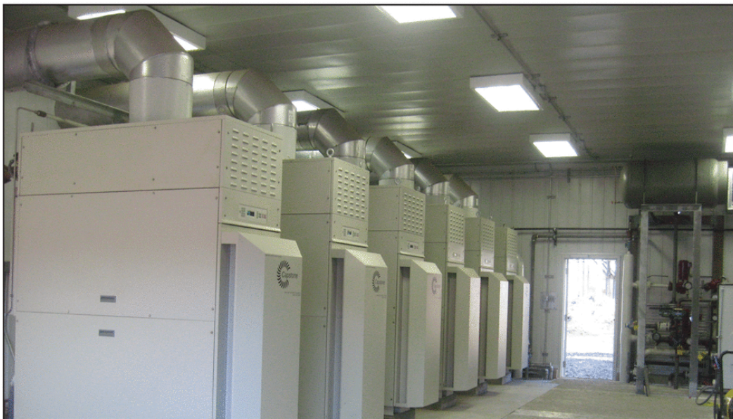
Basic Systems Inc. designed the expansion of this gas storage facility in remote north central Pennsylvania, U.S.A. Six Capstone C65 microturbines were initially installed to provide the additional power required for the expansion.
