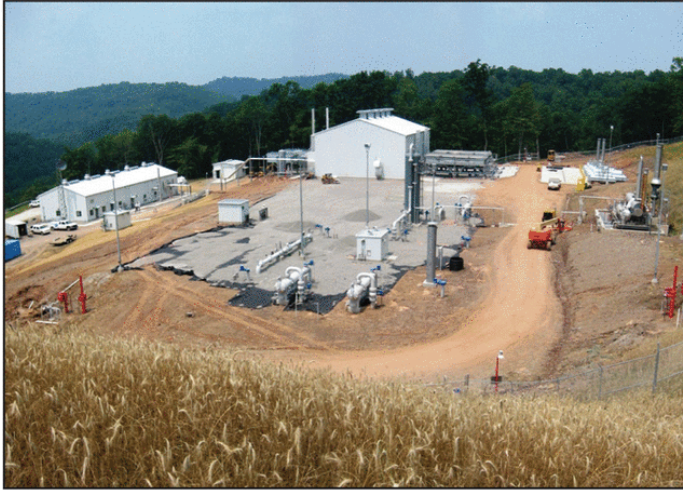
Electric power was not economically available at this greenfield natural gas storage facility in West Virginia, U.S.A. Basic Systems Inc.'s design included four Caterpillar G3608/Ariel JGC/6 compressor packages. Nine Capstone model C65 microturbines provide all the power for the site.
